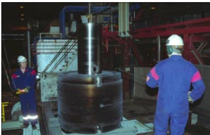
Shrinking of liner.
